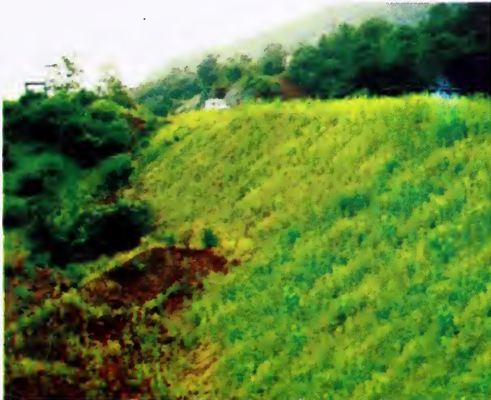
Fig. 13 Vegetation Growth after Application of 3-D Mats on Denuded Road Side Slope
