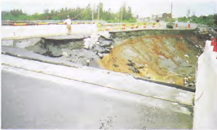
Fig. 5 Erosion Patterns – Severe Erosion of Approach Embankment by Flood Waters
