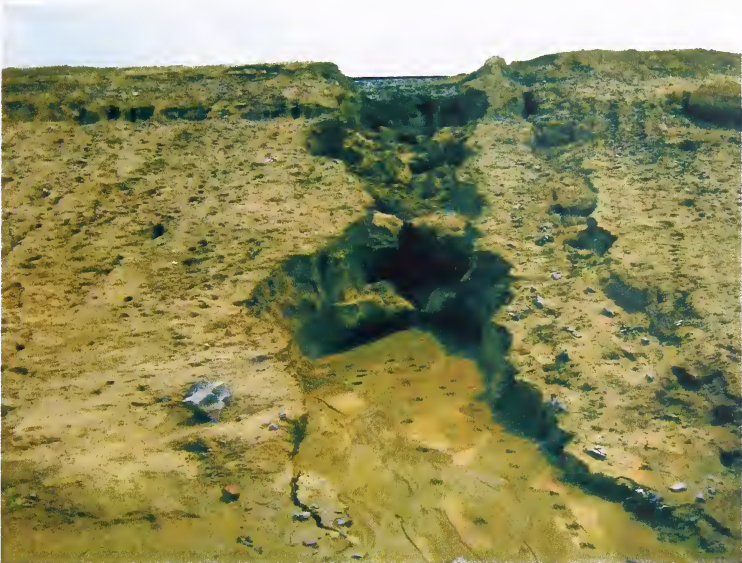
Fig. 3 Erosion Patterns – Deep Gully Formation in Embankment Side Slope
