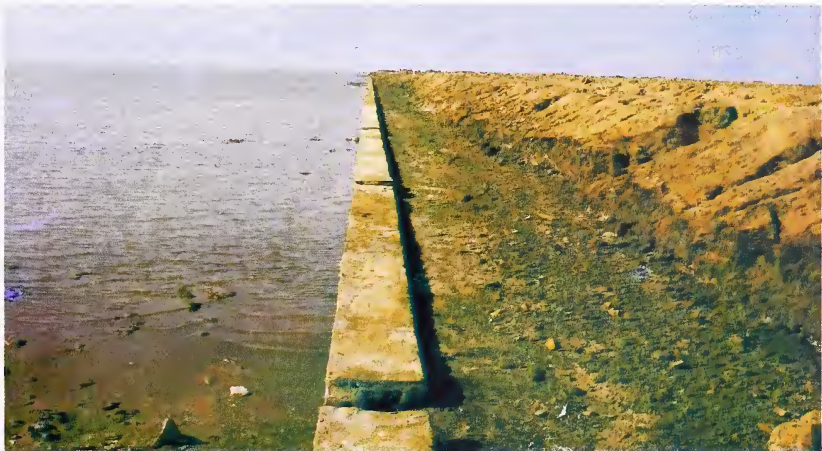
Fig. 4 Erosion Patterns – Embankment Toe Cutting by Flood Waters
