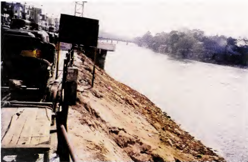
Fig. 33 : The Damaged Portion of Wharf Road Before Restoration
