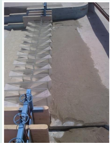
Under Sluices Gates Open Unequally
