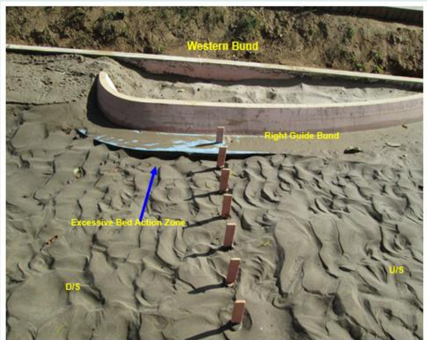
General View of Excessive Bed Action near Right Abutment
