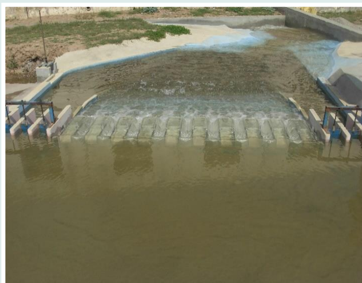
Running view of P. K. Weir from U/S with under sluice gate closed at 2500 m 3 /s discharge
