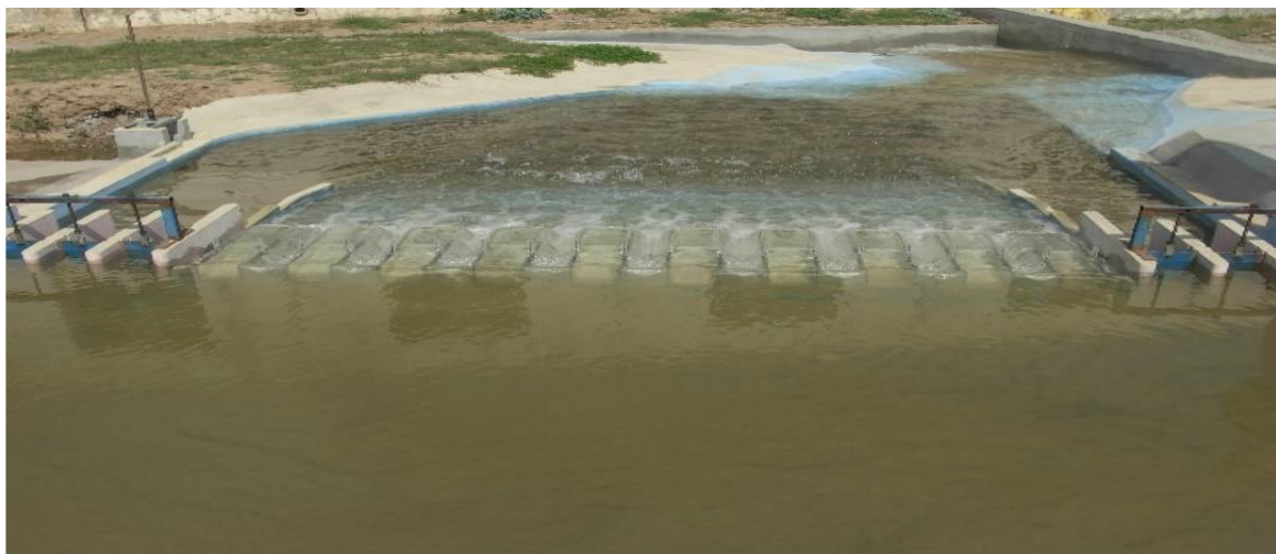
Running view of P. K. Weir from U/S with under sluice gate closed at 2500 m 3 /s discharge
